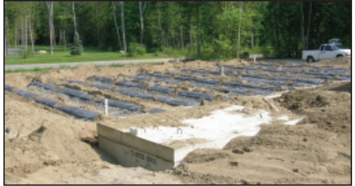
Septic tank and leaching bed.
